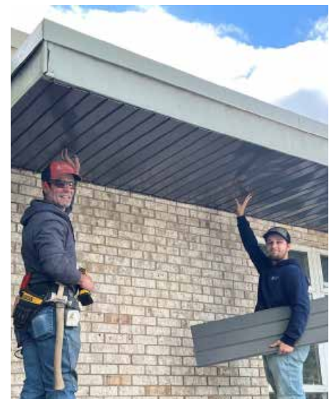
Scott Kerstetter and Kevin Knipe show off a new section of soffit at 350 Poplar Church
