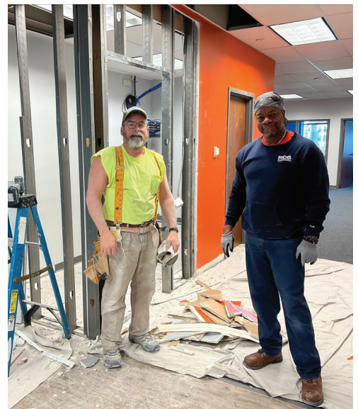
John Fry and Jack Cobb are shown here at 275 Grandview, where they are framing out walls for a new tenant.
