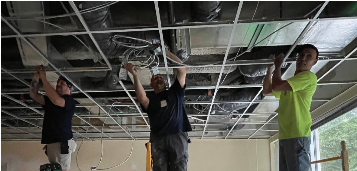
Jason Hare, Bob Kams and Greg Moyer of Capitol View Construction are installing a new ceiling grid and redirecting lighting and HVAC at Keystone Plaza
